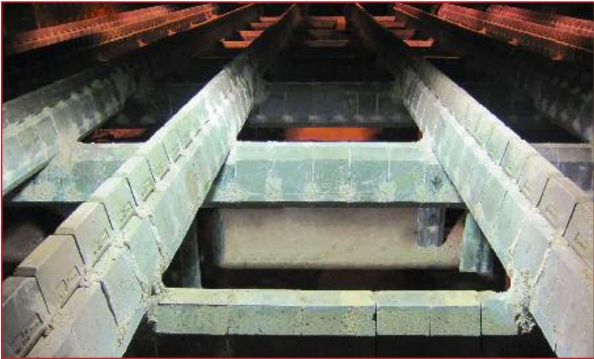
Skid system with new refractory shortly before recommissioning
